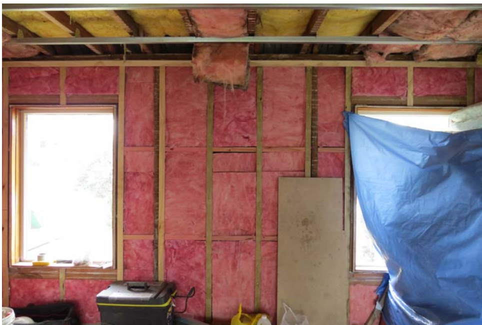
Figure 4: Wall insulation was installed and existing ceiling insulation topped up to cover the downlights
