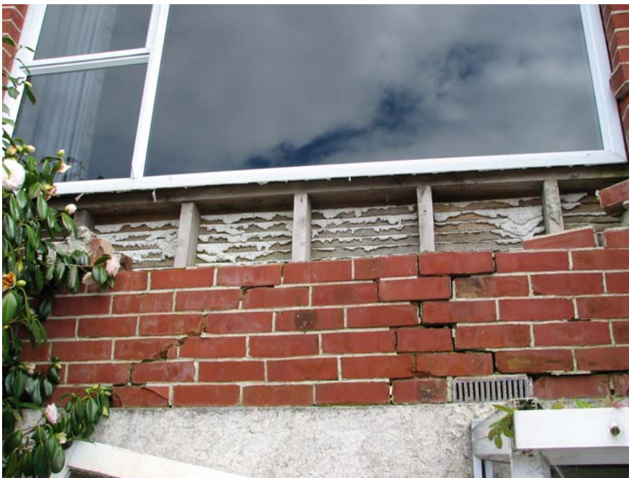
Figure 2: Cladding damage to Redcliffs 1
