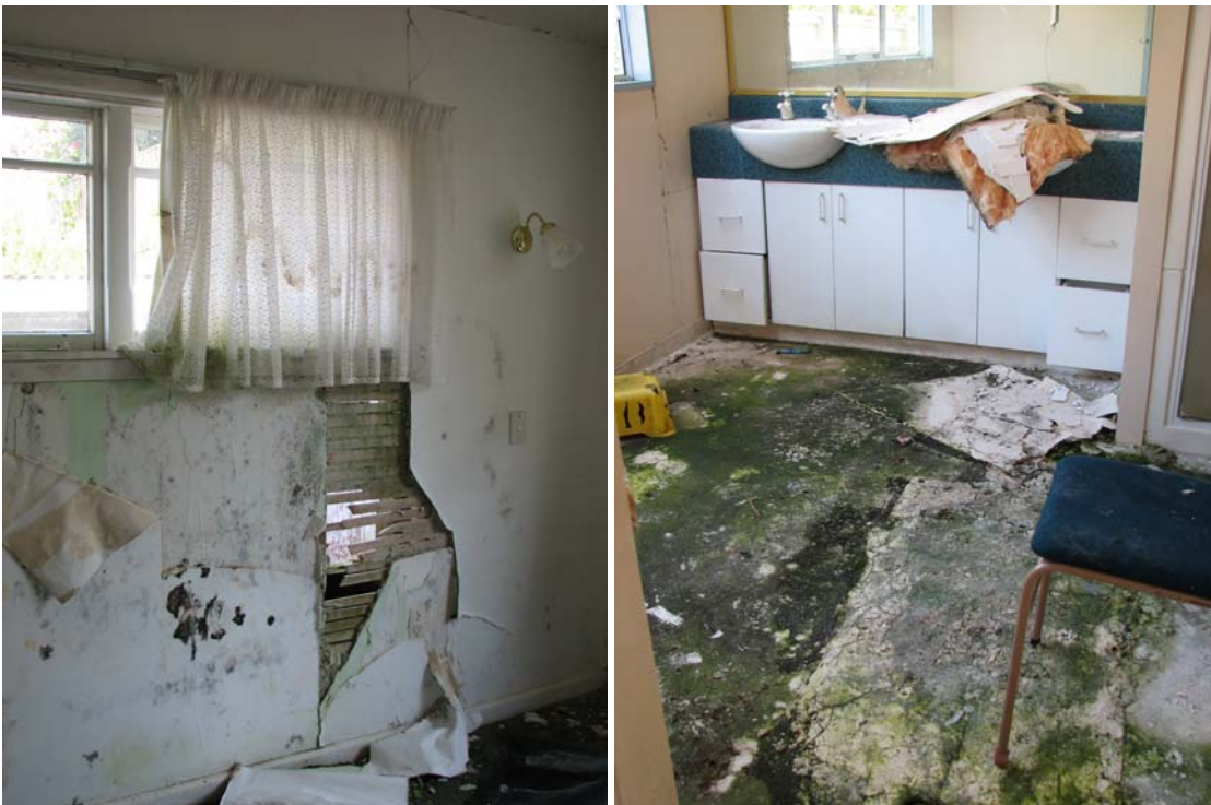
Figure 4: Internal water damage to Redcliffs 1 – damage was extensive throughout the house
