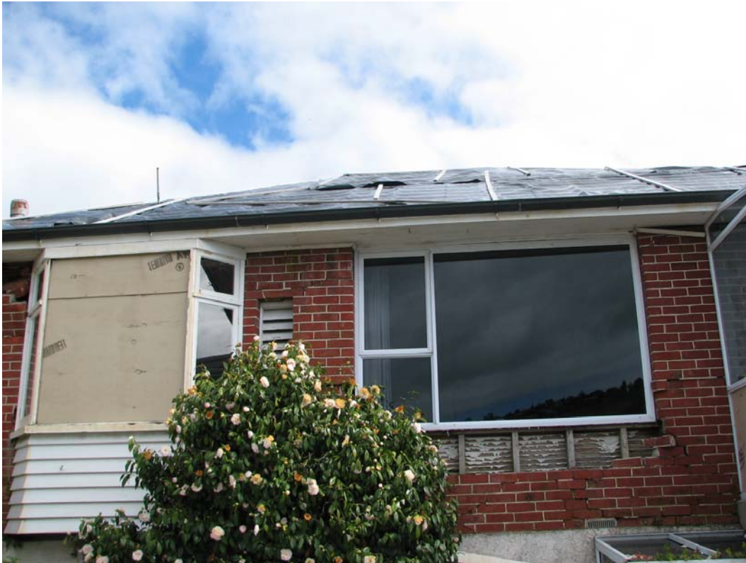
Figure 3: Roof and window damage to Redcliffs 1 with temporary weatherproofing
