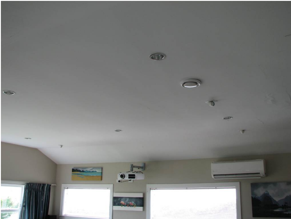
Figure 2: Ceiling damage to Mt Pleasant 1
