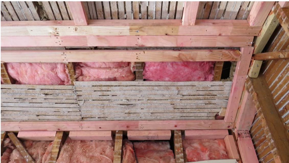
Figure 6: Lath and plaster ceiling and wall linings were not completely removed so insulation had to be fitted where possible.
