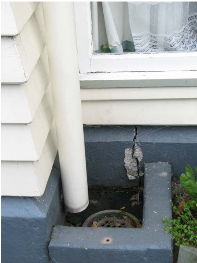
Figure 2: Earthquake damage to Somerfield 1 ring foundation
