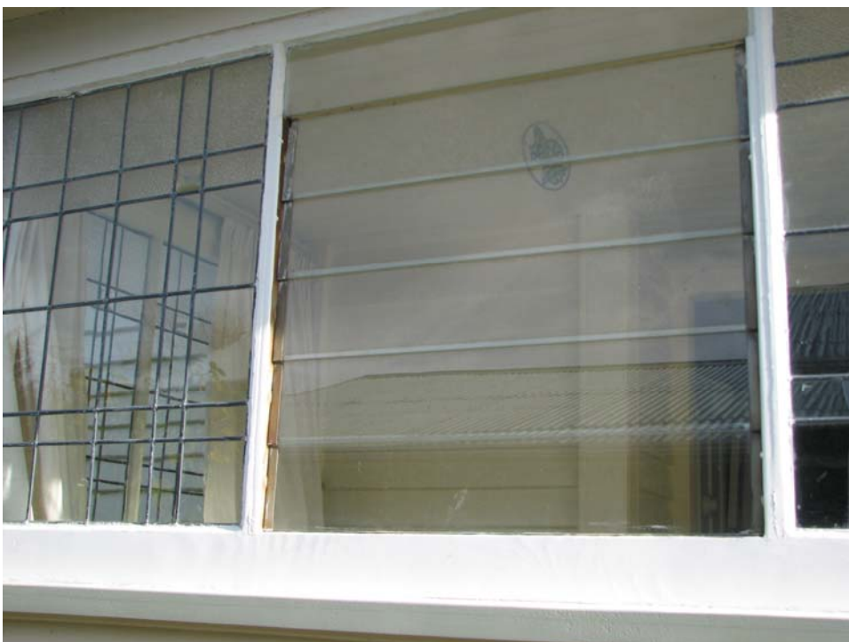
Figure 4: Louvre window in sun porch. This was causing significant draughts but the homeowner didn't want it replaced.
