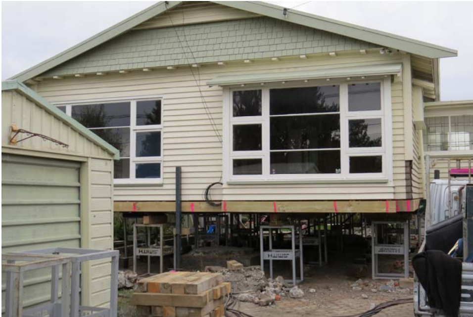
Figure 3: The house was lifted up for foundation repair – enabling access to install underfloor insulation and a ground vapour barrier in Somerfield 1
