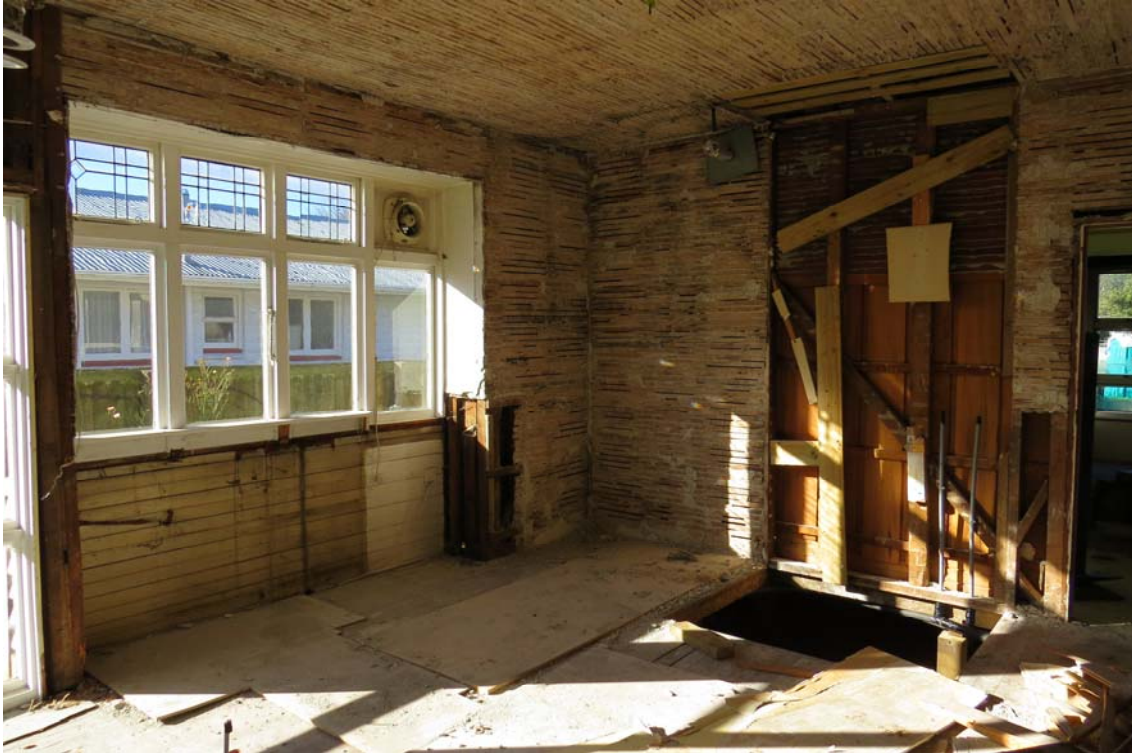
Figure 6: Lath and plaster linings were replaced with plasterboard as part of the repair, enabling wall and ceiling insulation installation
