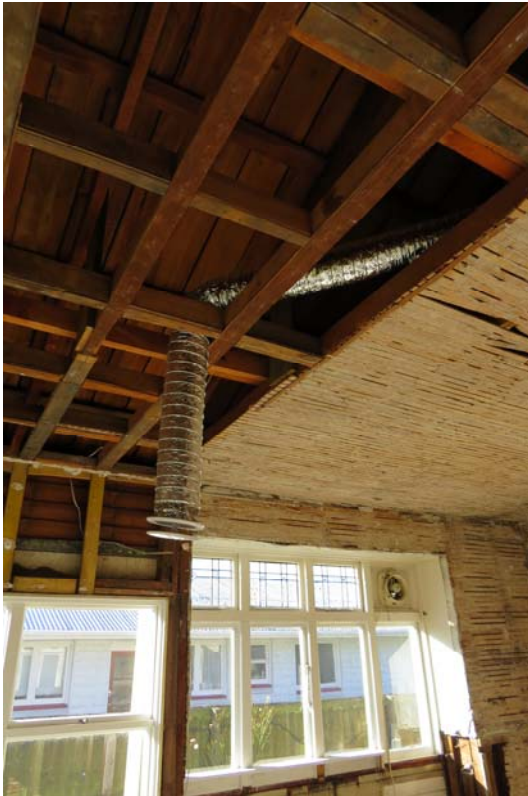
Figure 5: A positive pressure ventilation system had been installed by the homeowners to try and reduce the dampness in the house; however, mould and condensation were still prevalent
