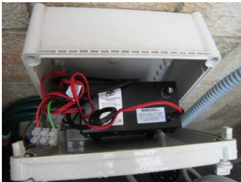
Figure 4: AC/DC Transformer for grey water system
