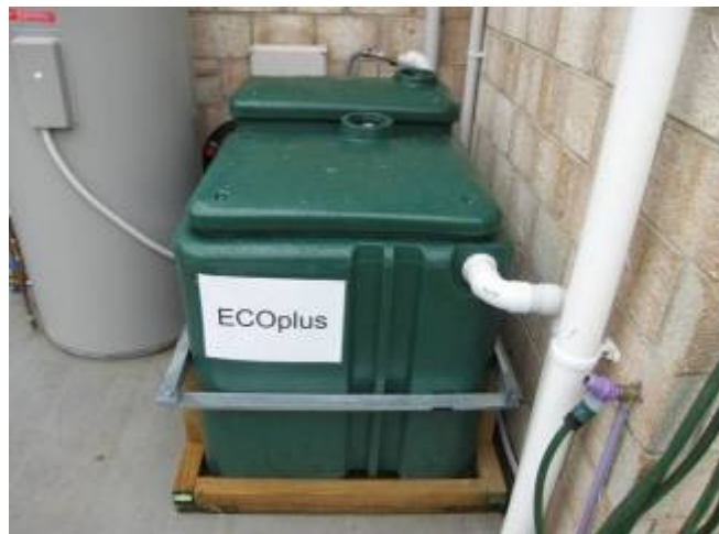
Figure 3: Eco-plus grey water system
