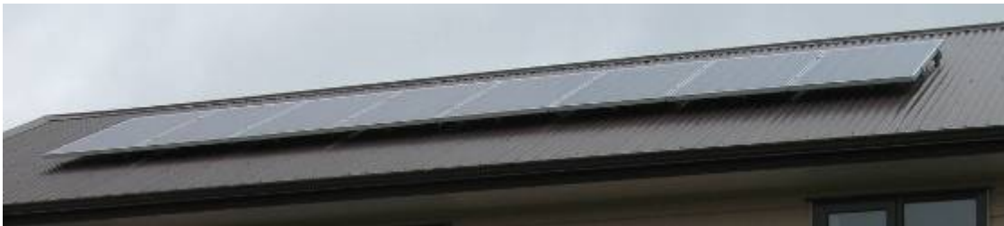
Figure 1: PV panels on the NWW facing roof side
