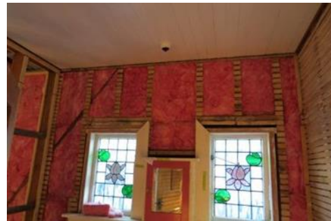
If your linings are being removed and replaced, wall insulation can be added from the inside.
