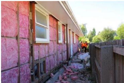
If you are having cladding replaced, wall insulation can be added from the outside.
