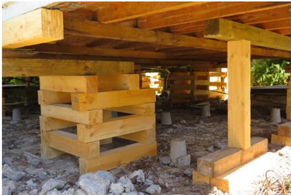
An older house lifted for pile replacement. You can see the original piles offered little space for installing either underfloor insulation or a ground moisture barrier.
