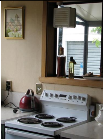
An example of ineffective ventilation – too far from the stove and not covering the full area. These types of ventilation are also often draughty when not in use.
