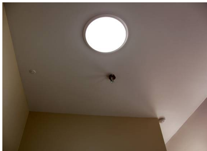
A Solatube lights the kitchen in the Waitakere NOW Home
