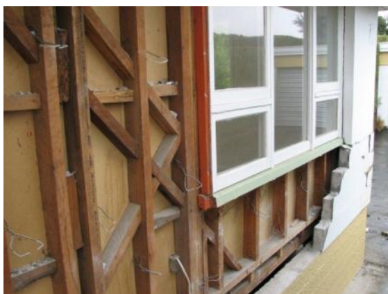
Original 1960's construction without wall insulation or building wrap uncovered as veneer removed.
