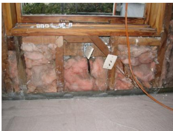
Poorly-fitted fibreglass batts installed in 1970s lounge renovation with no building wrap between insulation and veneer
