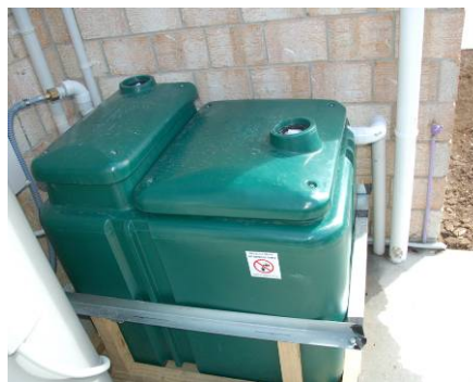
The EcoPlus greywater system
